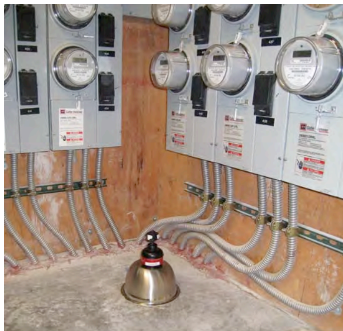
Figure 4 E-PERM Slab Emanation with room air measurement
