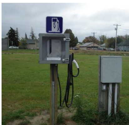
Level 2 EV Charger.
