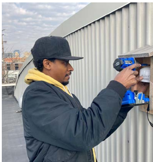
John Dandridge, NHBP DPW Maintenance Technician, installs a PurpleAir monitor at the Tribe's northern health office in Grand Rapids, MI.
