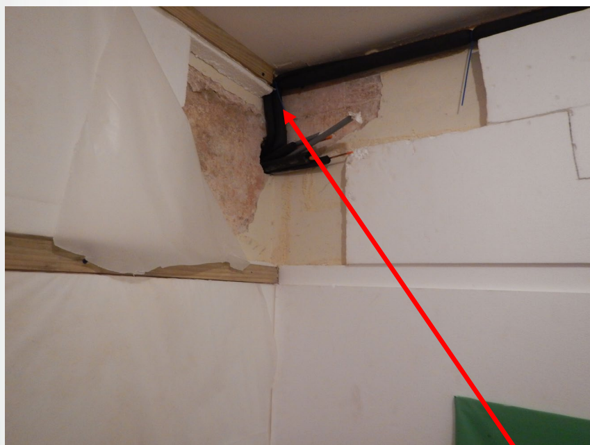
Identified radon gas entry point in home with >20 pCi/L levels
